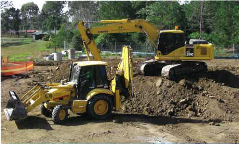
GW Civil's latest WB97R-2 backhoe, with one of its PC200-7s. The company opted for Komatsu backhoes based on operator preference following a competitive demonstration.
