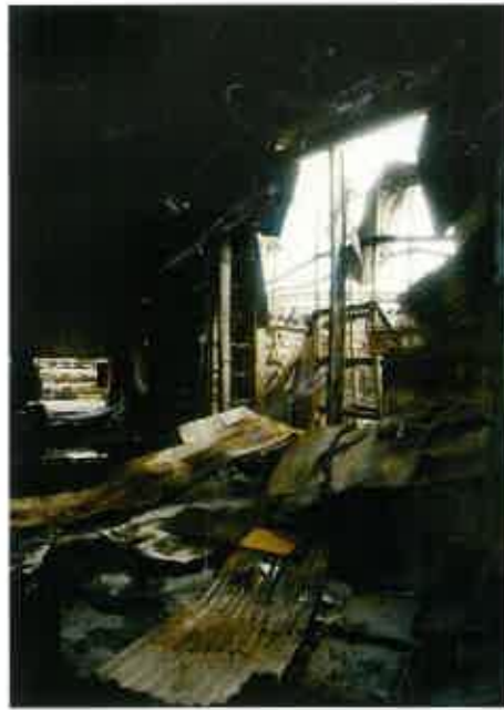
Down but not out. Just some of the damage caused during the fire.
