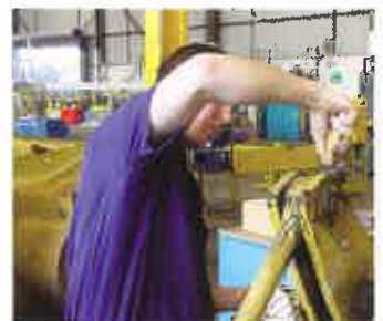
Use a scraper to clean off the worst of the dust and dirt that's built up around a joint...
