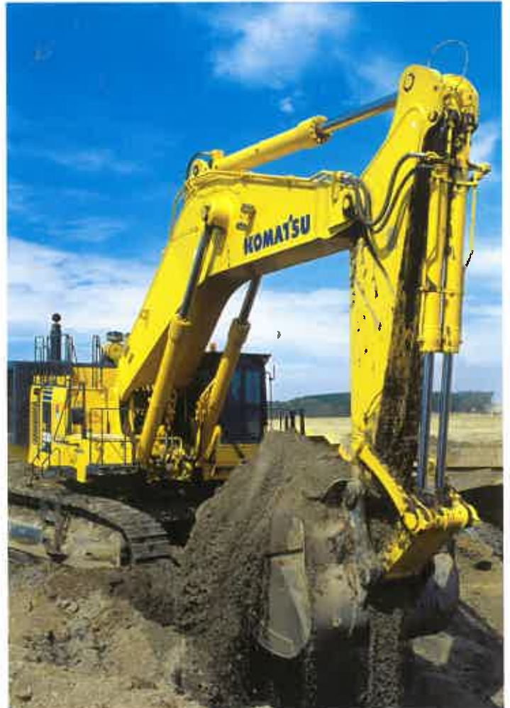
RTL's two new PC1250-7 excavators are giving significant increases in productivity over their predecessor machine.
