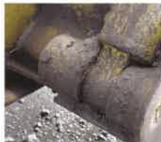
A leaking hydraulic cylinder, combined with poor joint cleaning and greasing practices just means more opportunities for contamination to enter the system.
