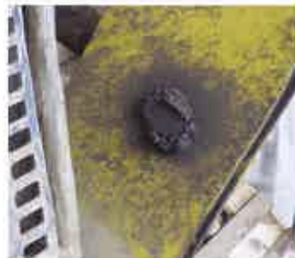
This is a grease nipple which hasn't been cleaned properly for a L-O-N-G time.
