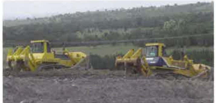
Two generations of Komatsu dozers working together: D375A dozers reshaping an overburden dump at Bulga Coal.
