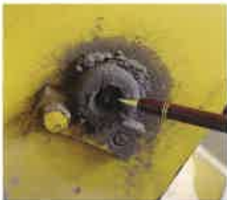
Excess grease around the nipple attracts dust and dirt which can get into the joint, shortening pin and bush life.
