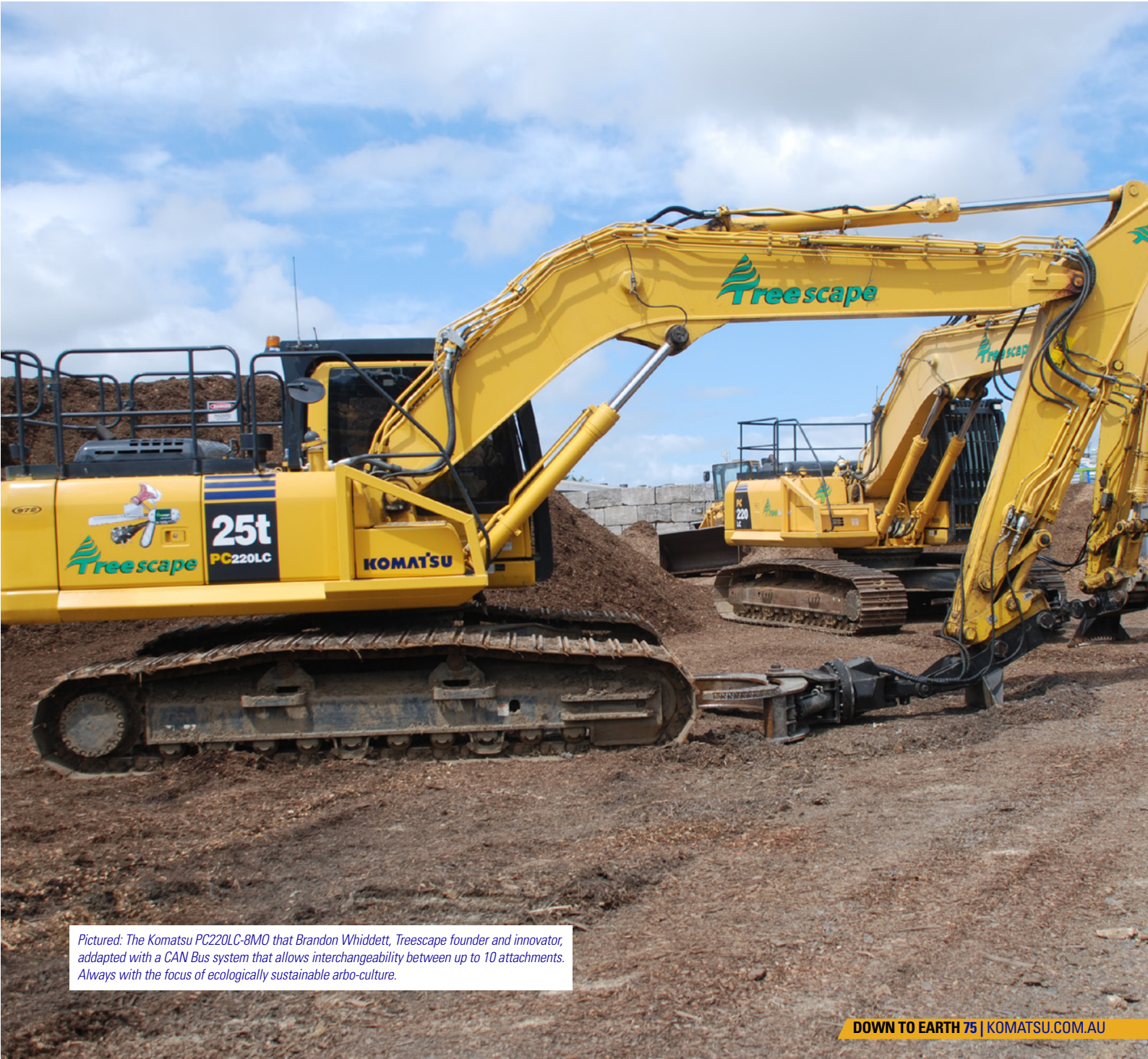
Pictured: Treescape and Komatsu have developed a strong relationship over many years of doing business together.
