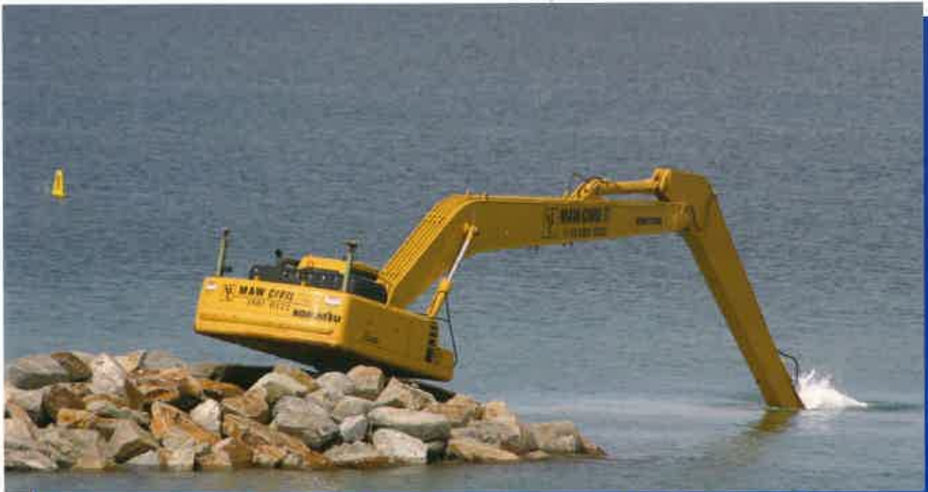
The dual features of the PC400-6 and Topcon's GPS are saving time and money for Maw Civil
