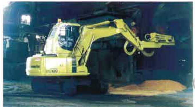
The PC120 at work in the Kalgoorlie Nickle Smelter.
