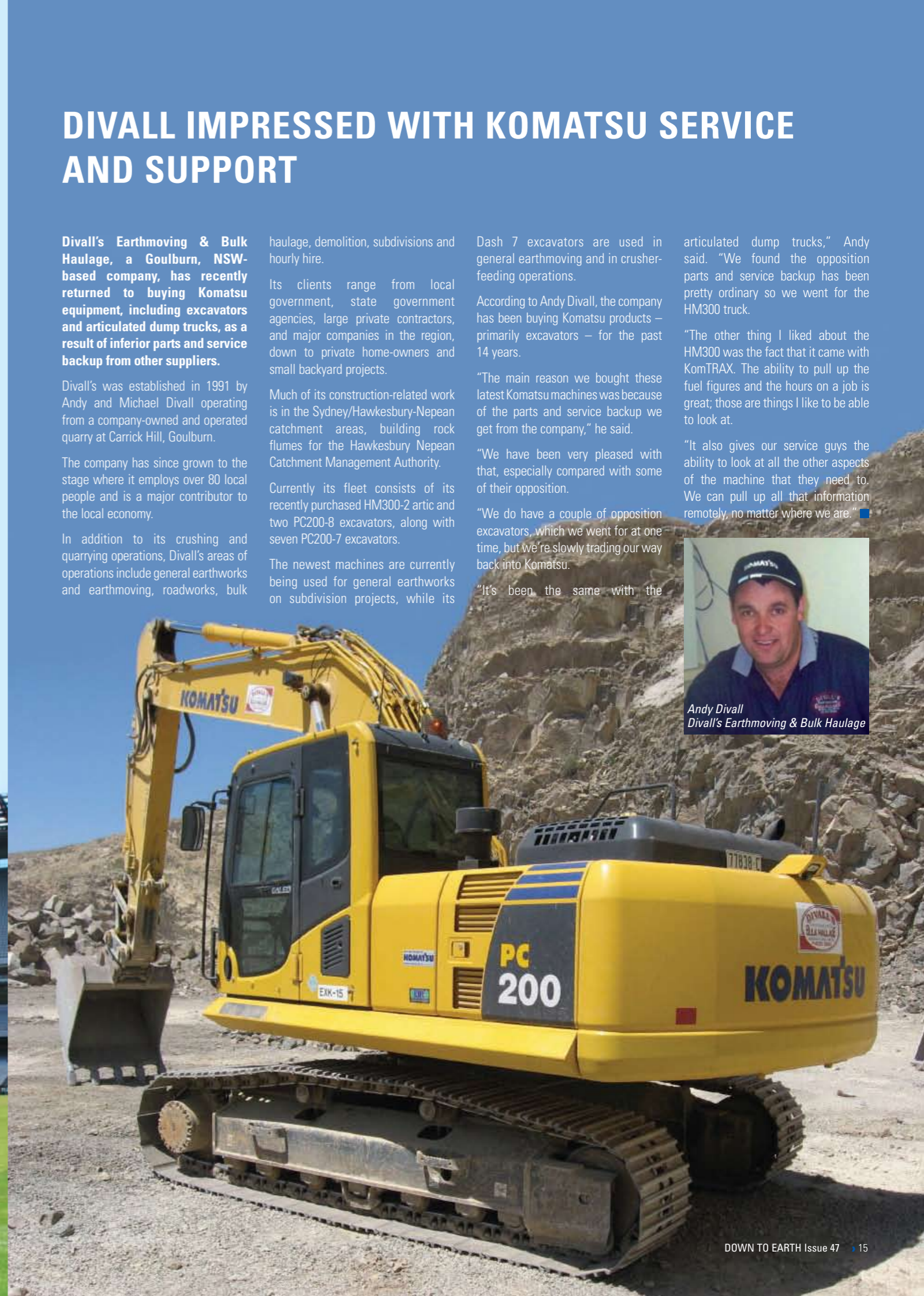
Pictured: The PC78UU is used to dig about 5mm excavated slots for the wicket tables at the Melbourne Cricket Ground each year at the beginning of the cricket season.
